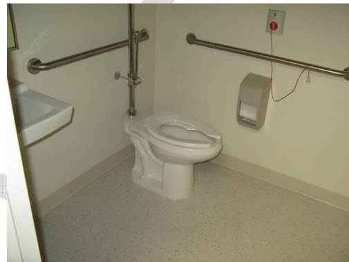
Patient Toilet Post-op flush control 50" AFF
